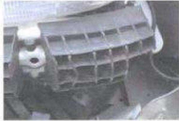
Damaged Core Fins
